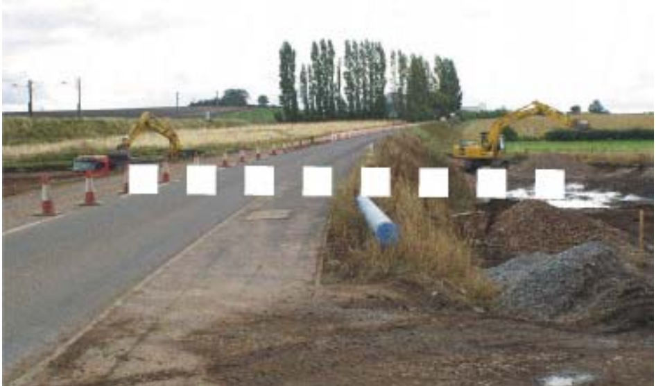
Approximate position of Lichfield Canal culvert underneath new roundabout (photo by Bob Williams).
