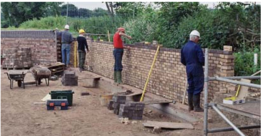
WRG BITM laying the top courses of the towpath back wall in the garden (Photo by Phil Sharpe)
