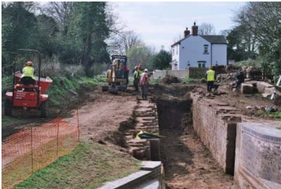
The excavated chamber of Lock 24 at the end of the Canal Camp (Photo by Phil Sharpe)
