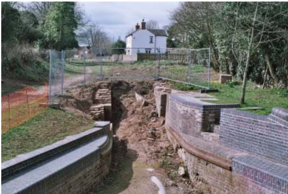
The partly exposed Lock 24 before the Canal Camp in April (Photo by Phil Sharpe)
