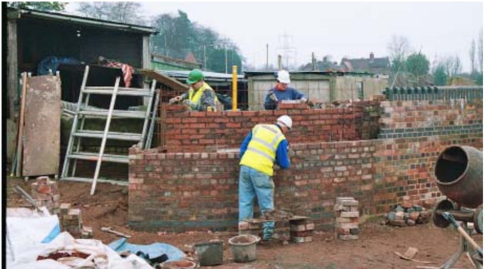
Brian and London WRG raising the offside top wing wall at Lock 26 Tamworth Road (Photo by Phil Sharpe)
