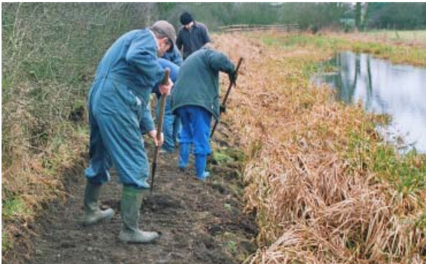
Denis and crew widening and levelling the Hatherton Canal towpath near Oak Lane (Photo by Phil Sharpe)
