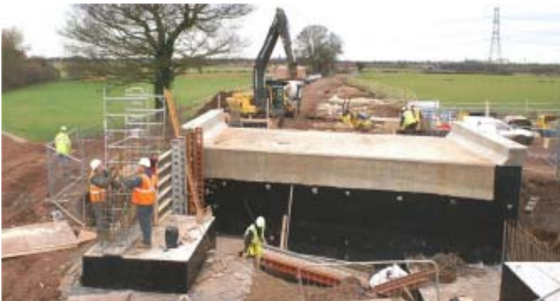
Forming foundations for wing walls at Cappers Bridge on 15 December (photo by Bob Williams)
