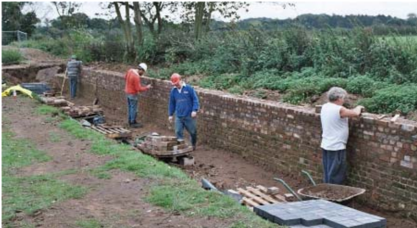
Trust and London wrg volunteers rebuilding the towpath wall (Photo by Phil Sharpe)
