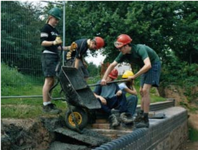
Wrg Canal Campers backfilling the wall with concrete at Lock 24 (Photo by Phil Sharpe)
