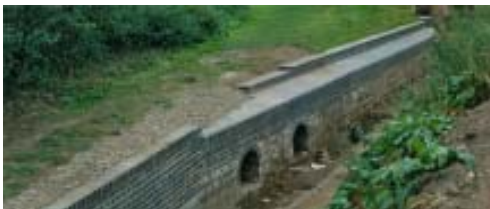
The completed towpath wall and landing stage at Lock 24 (Photo by Phil Sharpe)
