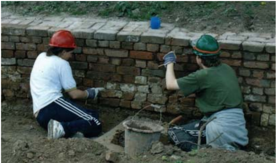
Canal Campers re-pointing the brickwork on the towpath wall (Photo by Phil Sharpe)
