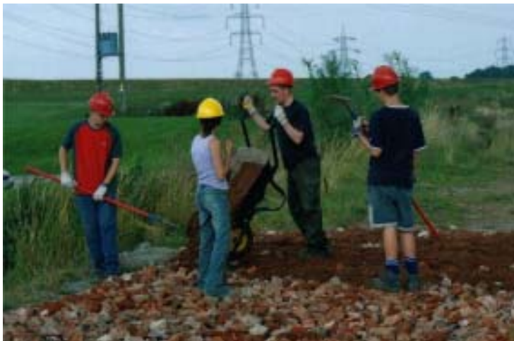
Canal campers reinstating the path at Darnford Lane with brick rubble and sand (Photo by Phil Sharpe)
