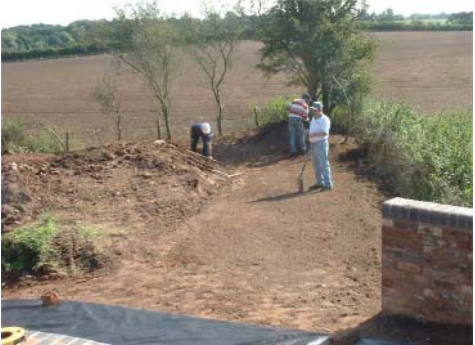
The Land Rover 'corporate citizenship' scheme supplied teams of 5 or 6 employees for 2 days a week over a 4 week period, Their main job was to level and landscape the 'triangle' area below Lock 25 and to improve the access (Photo by Bob Williams)
